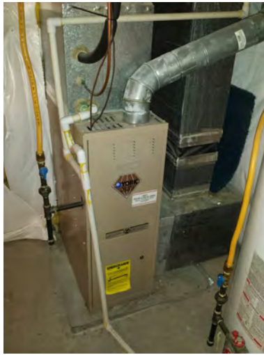
HVAC and Hot Water
