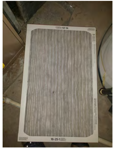
HVAC and Hot Water
