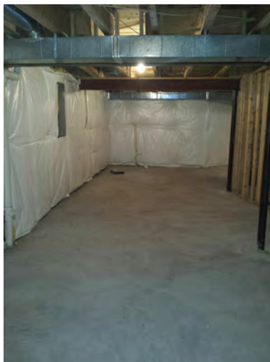
HVAC and Hot Water
