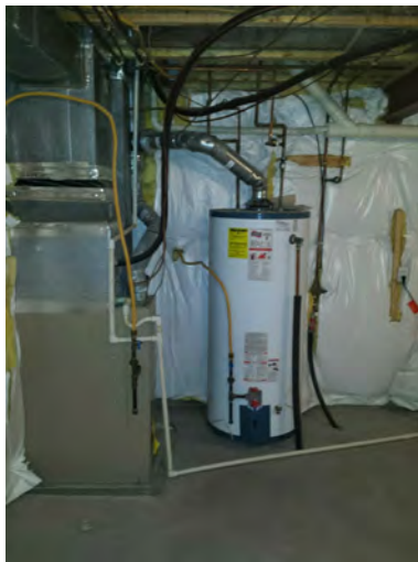
HVAC and Hot Water
