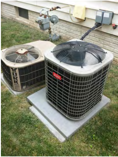
HVAC and Hot Water
