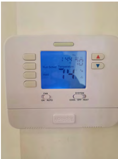
HVAC and Hot Water
