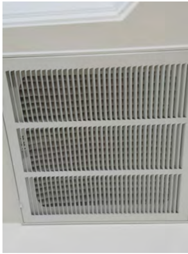
HVAC and Hot Water
