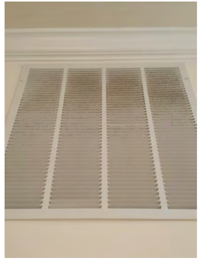
HVAC and Hot Water
