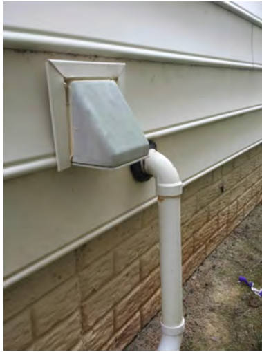
HVAC and Hot Water
