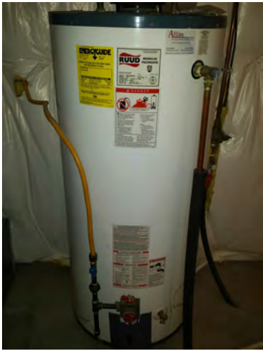
HVAC and Hot Water
